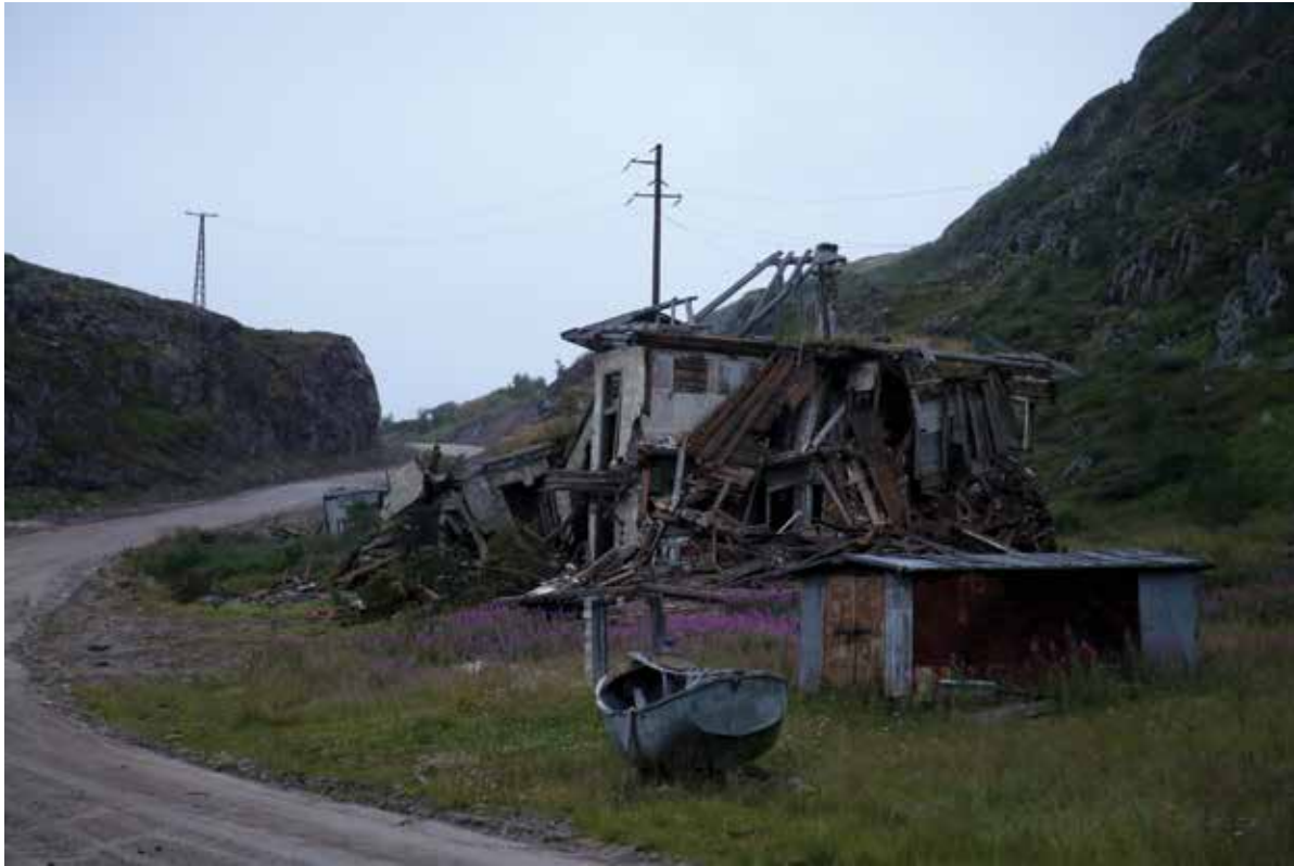
The All Infrared Line , photo, 2014. Collapsed building in Teriberka village.
